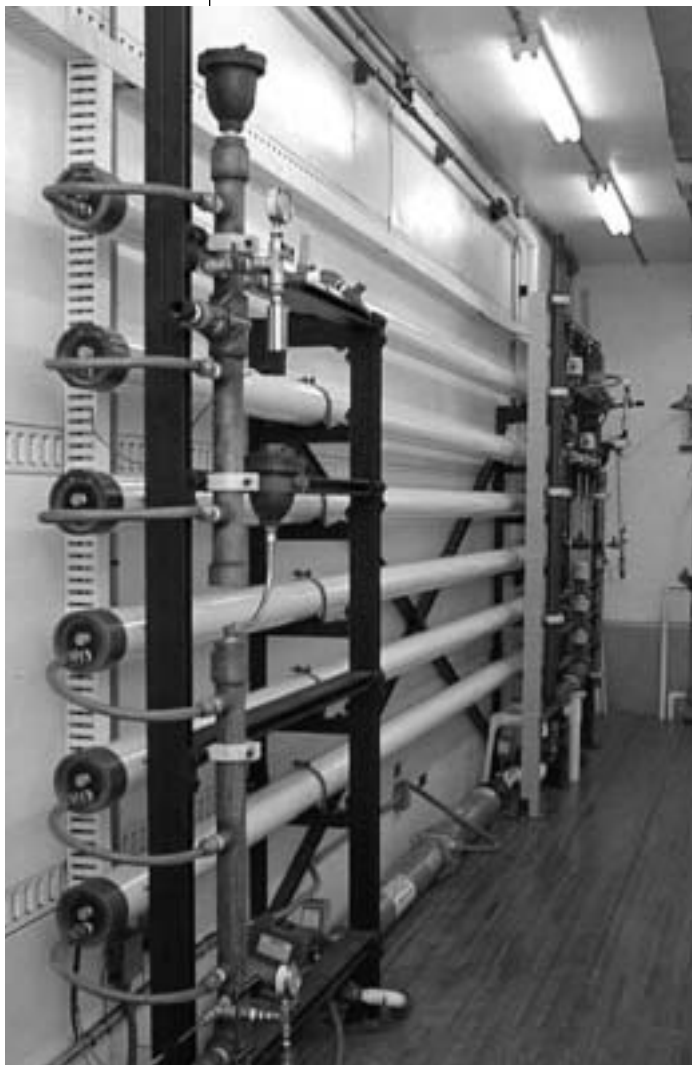
Figure A.: Pilot Trailer Equipment
